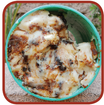
Figure 2: FOG is the most common cause of pipeline blockages.
