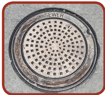
Figure 4: Manholes can be a common source of inflow in a system.
