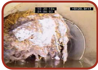
Figure 1: Root mass which entered the pipe line from a lateral.
