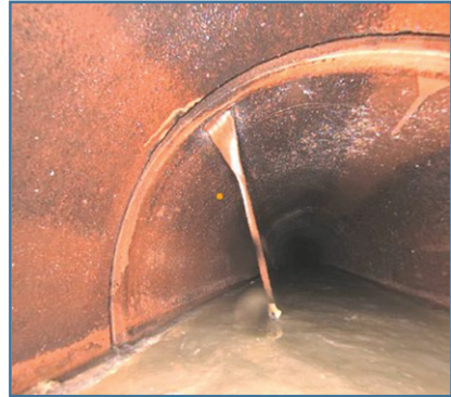
Figure 29: CCTV image of polyurethane gasket overpour
