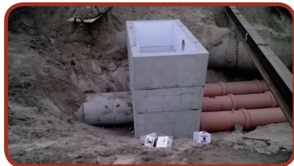
Figure 9-2: Triple barrel VCP constructed under existing 72-inch conduit into a junction chamber
