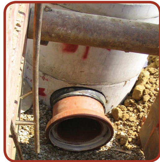
Figure 9-3: Short stubs and/or flexible manhole connections should be used to provide flexibility
