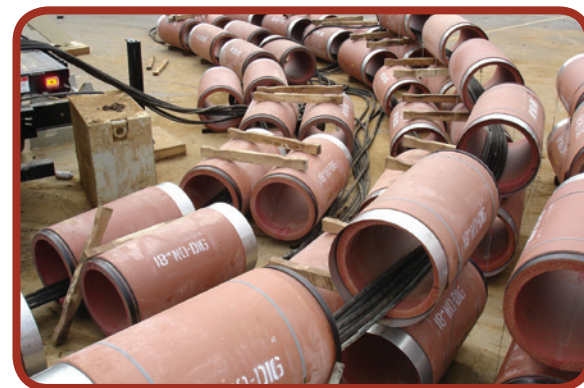
Figure 8-5: Jacking pipes staged at the launch pit on a pilot tube project utilizing a powered cutter head.
