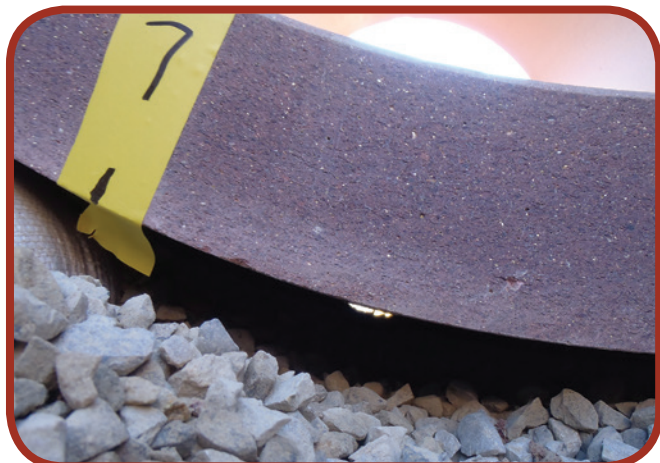
Figure 6-11: In testing, daylight was visible on the other end of a length of pipe.
