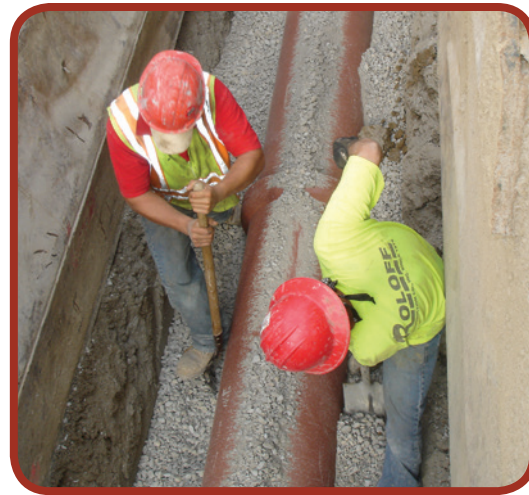
Figure 6-8: Shovel-slicing the bedding material into the haunches of the pipe is essential if the total load factor is to be realized.
