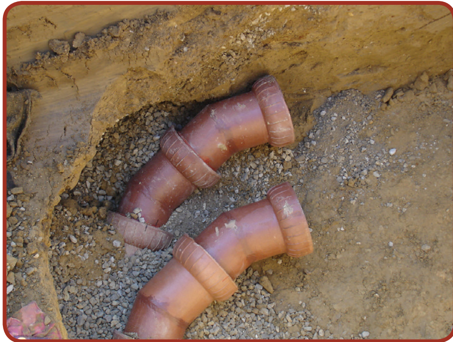
Figure 10-1: 6-inch VCP curves connected to the sewer main via wye fittings
