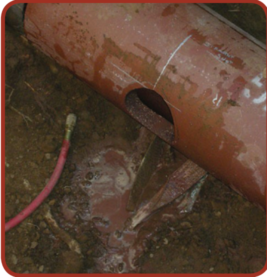
Figure 10-4: Hole cored in clay jacking pipe to reconnect a lateral following a pipe burst.
