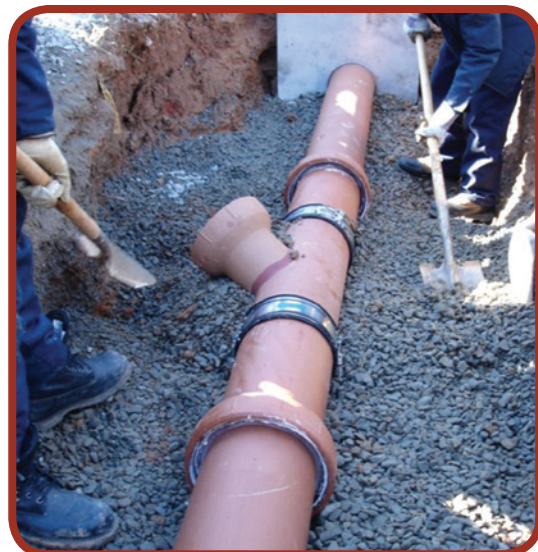
Figure 10-7: Wye fitting for lateral service connection to main line made using shielded rubber couplings.
