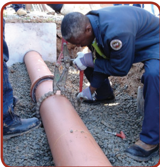
Figure 10-6: Cutting out a section of main line to insert a factory made, plain-end wye fitting.
