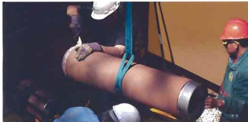
Top to bottom: Pipe Bedding Test Equipment and Preparing Microtunneling Pipe for Insertion
